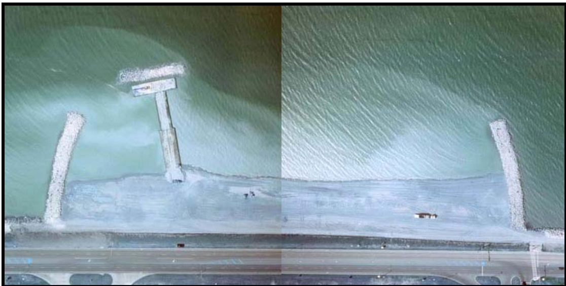
Figure 2. Mid-construction aerial view taken during construction of west DBW, 07/28/2001 (Lanmon Aerial Photography, Inc.).
